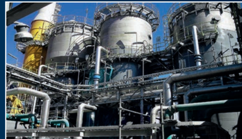
Absorbers, process basins and pipes are e.g. lined with rubber and additional bricks in non-ferrous metal extraction and acid production plants.
