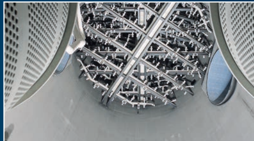
Flue gas desulphurization scrubber – Steuler rubber linings for very high chemical, thermal and mechanical requirements.
