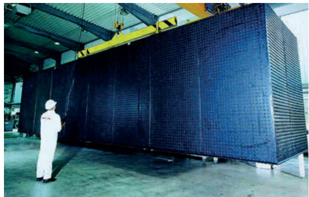
Above picture: A hydrochloric acid pickling plant is renovated using a pre-fabricated Bekaplast™ immersion tank accommodating contents of over 100 m³ thereby saving lots of time.
